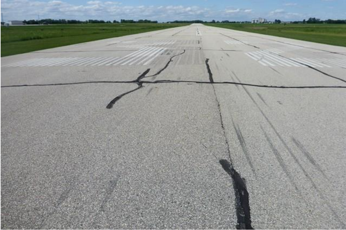
DXX RY1432 001 prior to slurry seal (PCI = 63, 6/2/2016)
