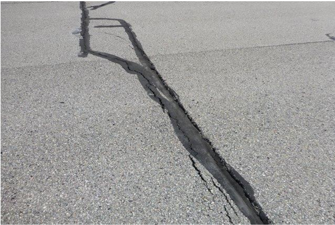
DXX RY1432 001 prior to slurry seal (PCI = 63, 6/2/2016)
